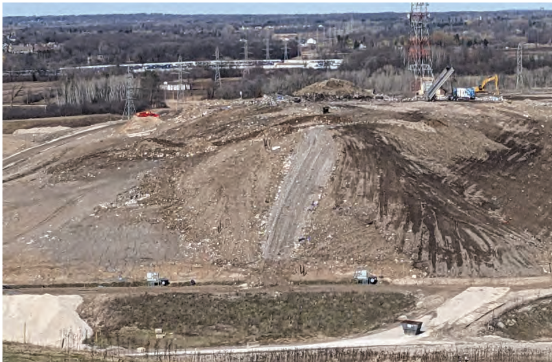
North Expansion West well covered; new cover being improved on East side
